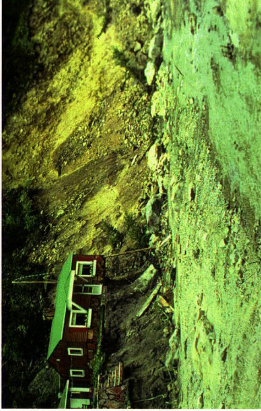
ID. BIG THOMPSON CANYON FLOOD no. 17ct! House precariously undercut by lateral scour, Big Thompson River 1/4 mile below Glen Comfort, Glen Haven Quadrangle. Landslide to right in background caused by undercutting; a house was carried away at that point. River flows toward observer. Aug. 13. 1976.
